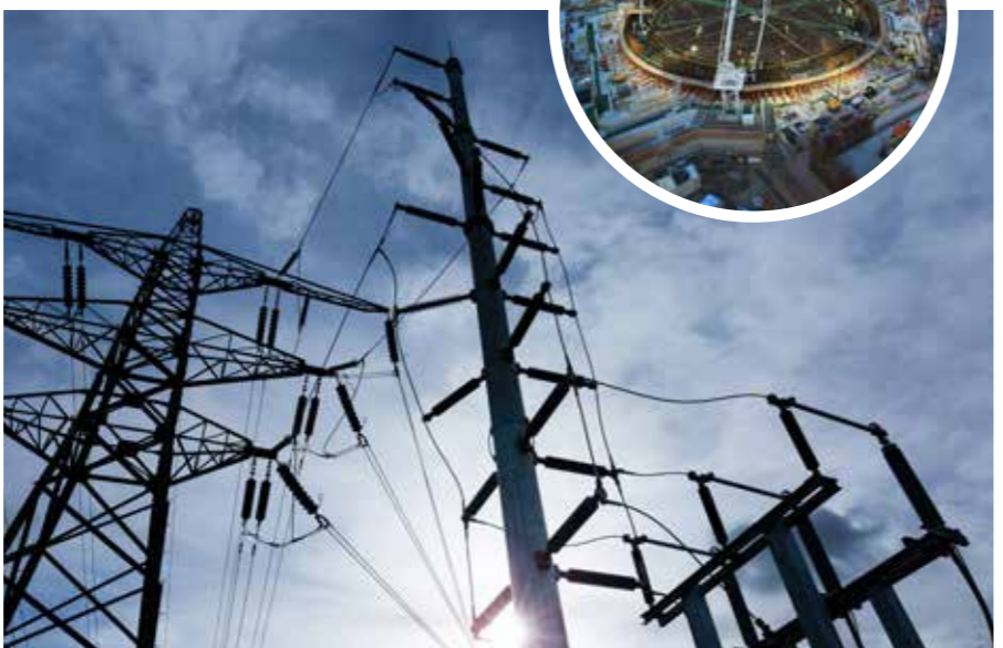
▲ Point of Connection Mast - POC-MAST™
